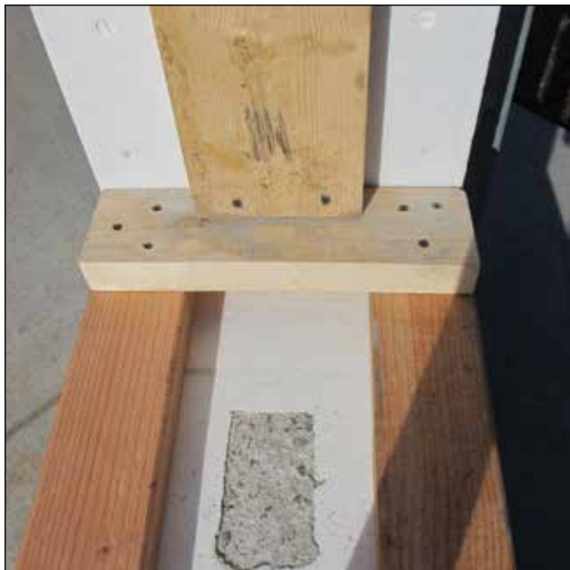
Figure 2.4 Corner bracing properly attached to lateral and longitudinal braces. Side braces attached to buck face.
