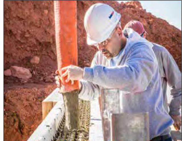
Figure 3.2.2 Pouring concrete into an ICF basement using a pump truck and flat hose.
