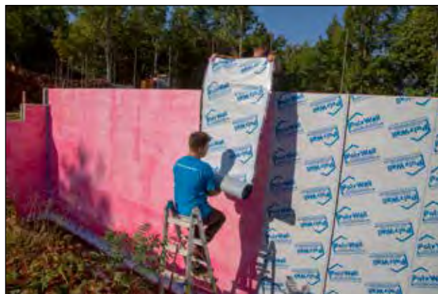
Figure 6.4.5 Poly-Wall Home Stretch Membrane is installed lapping seams at least 3" so water flows over the seam not against it.
