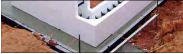
Figure 6.1.5 String lines used to ensure square and ICF form above corner forms locking corner in place until set.
