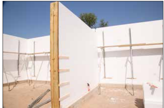
Figure 5.12.1 An end wall, properly bucked and strapped prior to installation of bracing & alignment system before concrete pour.
