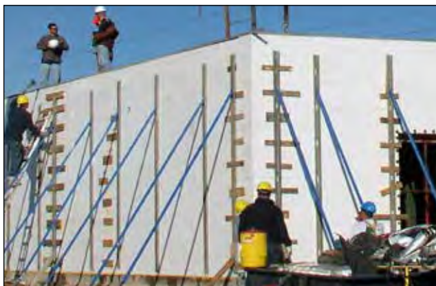
Figure 9.6.5 Ample Outer Bracing with "Scabs" on Non-Factory or Irregular Cut Joints (No Walk Boards)
