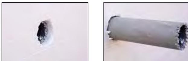
Figure 7.1.3 Cut small teeth on one end of the pipe sleeve and use to saw through the other side of the block to create a smooth opening.
