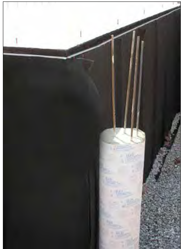
Figure 6.4.9 Basement with pier for footing above. This is done to prevent sagging of footing as the disturbed soil settles.
