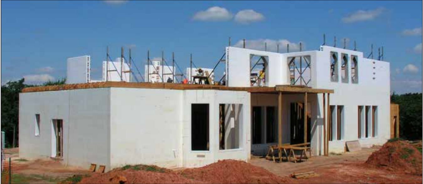
Figure 5.8.1 This partial second story has many openings, steps in height, bulkheads for wood frame attic, and is braced on the inside of the wall.
