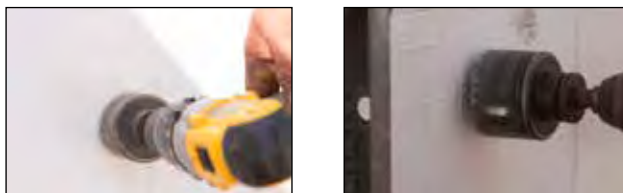
Figure 7.1.2 Drill hole the same diameter as the pipe sleeve to be used.
