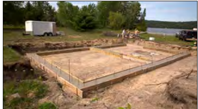
Figure 4.1.8 Place vertical rebar dowels with the correct height to join in the ICF wall.
