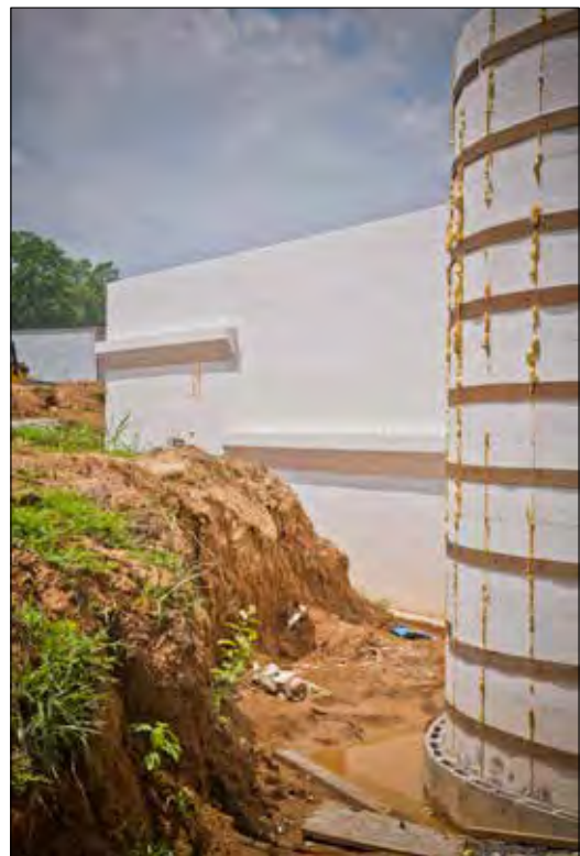
Figure 6.3.2 Brick ledge forms installed at varying heights to support masonry facade above grade.
