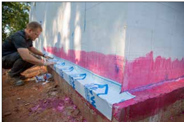
Figure 6.4.3 Installer placing a self-adhesive waterproofing membrane. Notice the 12" of membrane at the bottom of the wall sealing the footing to the wall.
