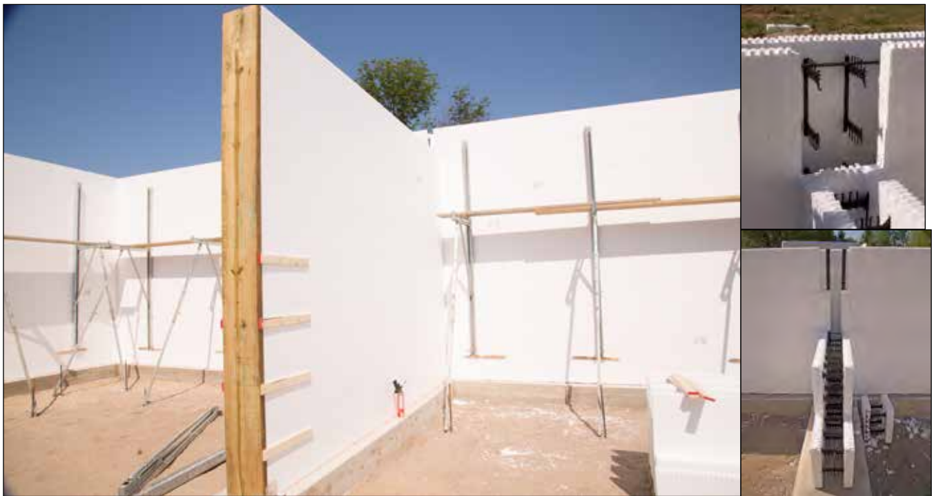
Figure 5.5.1 Intersecting Bulkhead wall with strapping. Figure 5.5.2 (top) Wall intersection opening cut. Figure 5.5.3 intersecting wall opening types.
