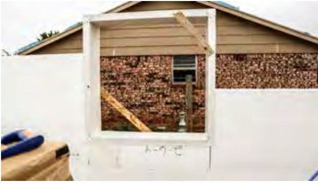
Figure 8.1.2 V-Buck ICF bucking placed into the walls. Notice cross-bracing on corners to ensure it remains square.
