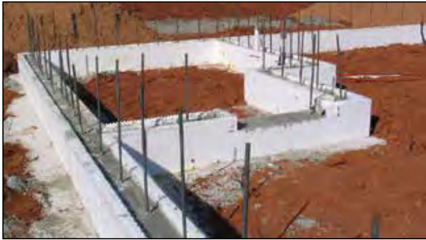
Figure 4.3.4 Wet set BuildBlock ICF stem wall. The first course is square, stacked, and poured. The site is now ready for the slab to be poured. Notice the rebar extending at least 24" vertically and the clean interlocks so the next course can be stacked.
