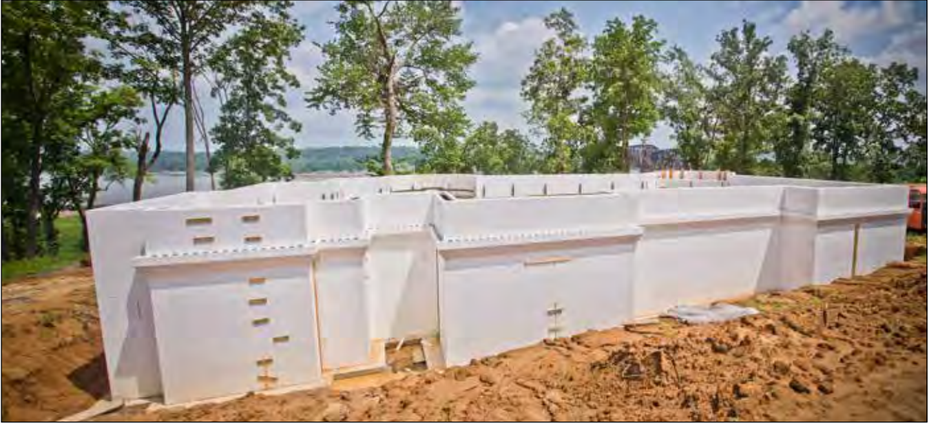
Figure 6.3.1 ICF walkout basement with brick ledge installed to support masonry veneer above grade.
