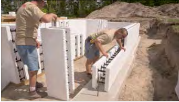
Figure 4.3.1 Stacking first two courses starting from a corner and working in a single direction.
