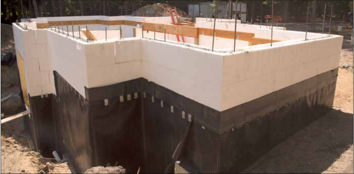
Figure 6.4.1 Below grade ICF walls with peel and stick membrane waterproofing applied and Air Gap barrier to prevent damage from backfill and provide hydrostatic pressure relief.
