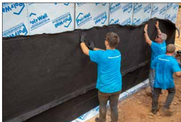
Figure 6.4.6 Arroyo Drain Board Waterproofing and air gap membrane is installed and brought to at least 1-foot above backfill level. Comply with local codes.
