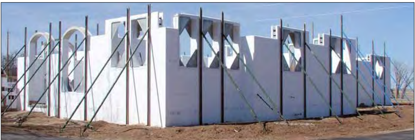
Figure 8.4.2 For larger openings than 3' wide, additional bracing and "bracing legs" (long 2x4 wood legs screwed to the vertical bucks and run to a base plate will help keep your openings straight and plumb during the pour..
