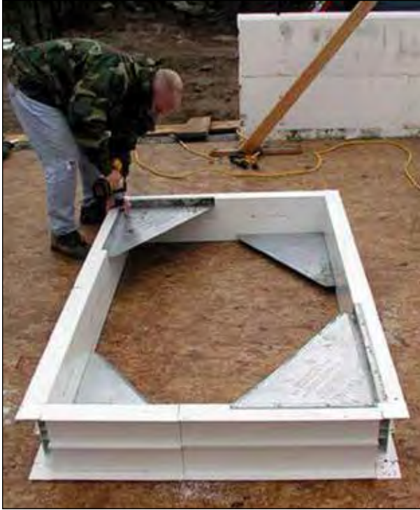
8.2.1 All bucks must be angle braced to keep them square and true.
