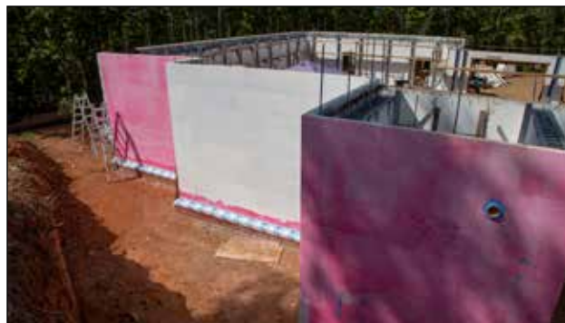
Figure 6.4.4 Detail strip attached along footing and corners. Walls partially primed for Home Stretch membrane installation. Membrane is attached to the ICF wall and sealed to the top of the footing.
