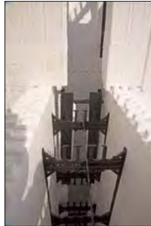
Figure 5.5.6 Intersecting wall opening with wire used to secure webs to intersecting block.
