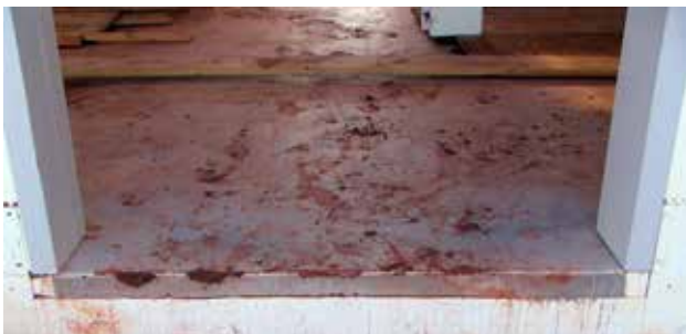
8.2.2 Note the concrete threshold poured to the outside wall edge. Bucking was properly braced during the pour to prevent any warping or cupping. Doors do not use bucking on the bottom of the door frame. Also notice the slab poured over the door threshold by cutting the block out 1-2" below the door height.
