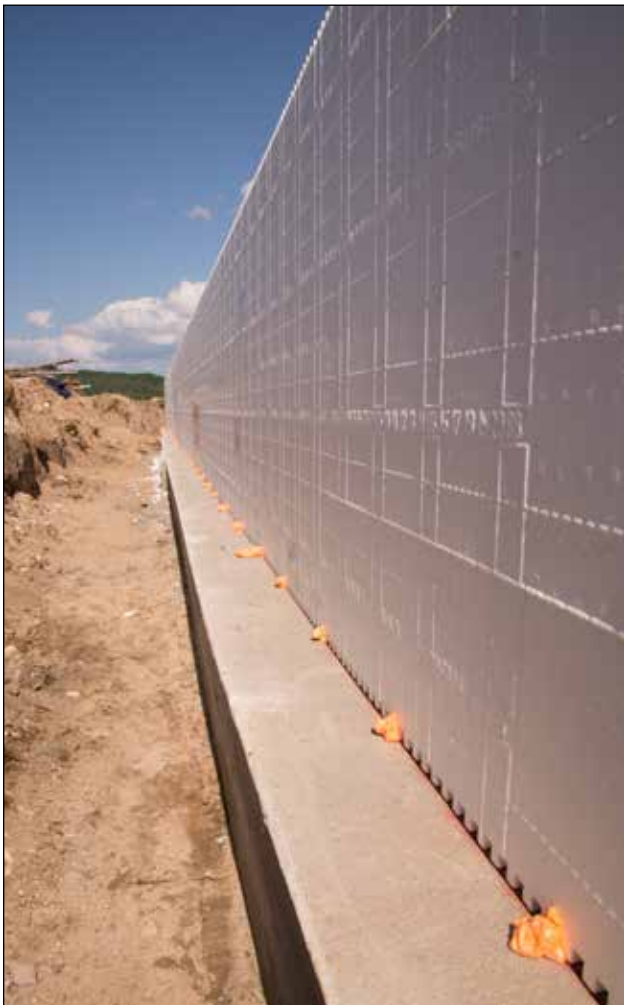
Figure 4.3.2 First two courses leveled and spot glued using foam adhesive. Use small amounts to prevent lifting the wall. Add additional adhesive after spot glue sets if desired.
