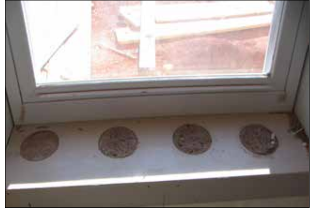
Figure 8.1.4 Fill holes cut into the bottom of a window. Ensure entrained air can escape when pouring a window to prevent any voids.
