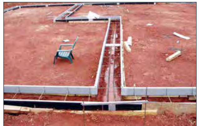
Figure 6.1.4 Form-A-Drain footing layout with rebar placed on chairs and Form-A-Drain Spacer Straps.
